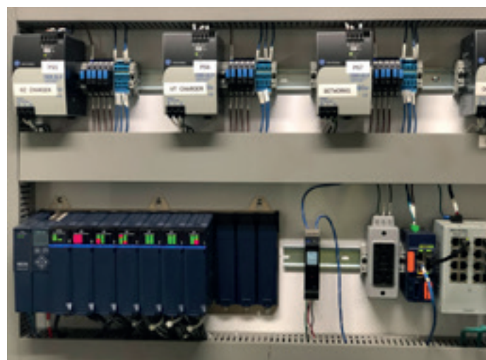
The RMC200 (lower left) in the new Maxi Mill control cabinet
